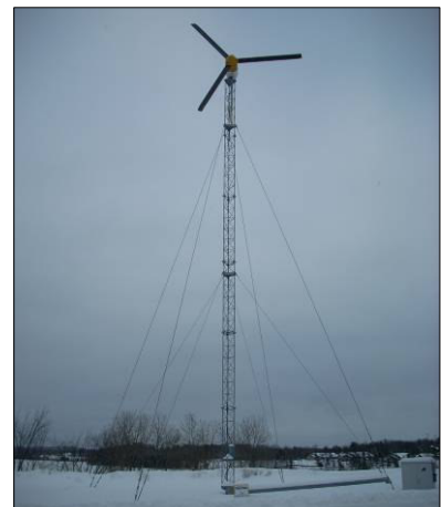
Wind Power Generator
